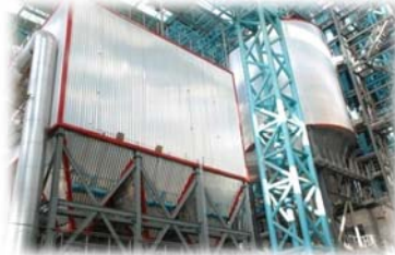
Fuel gas purification system
