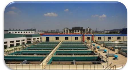
Landfill leachate treatment system
